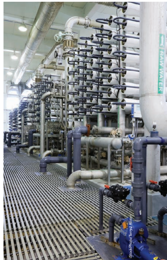
Filters in a reverse osmosis water treatment plant.
